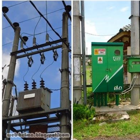
Gambar 5.9 Gardu distribusi jenis portal
